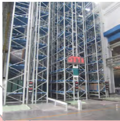
Automatic Storage and Retrieval System
