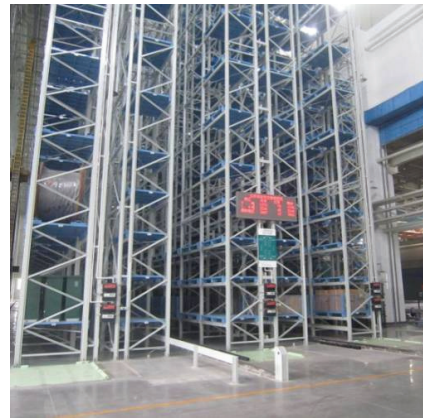
Automatic Storage and Retrieval System
